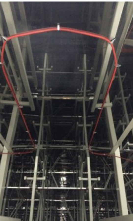
Optical fiber cable installation in the warehouse
