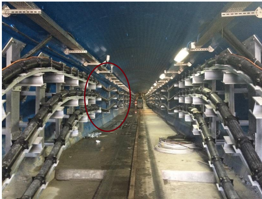
Power circuit through tunnel with sagging
