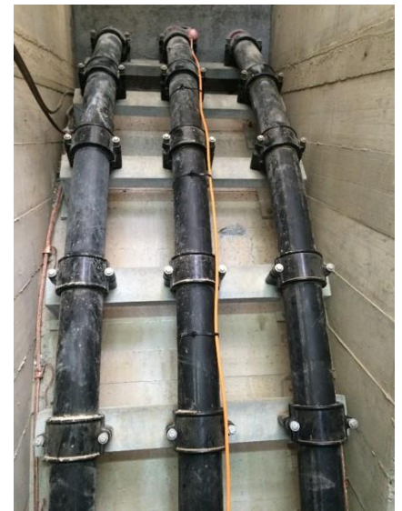
Central phase monitored
