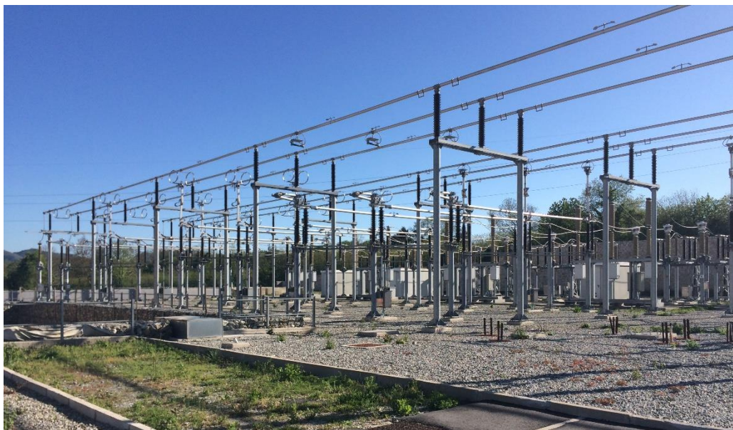
High voltage power cables
