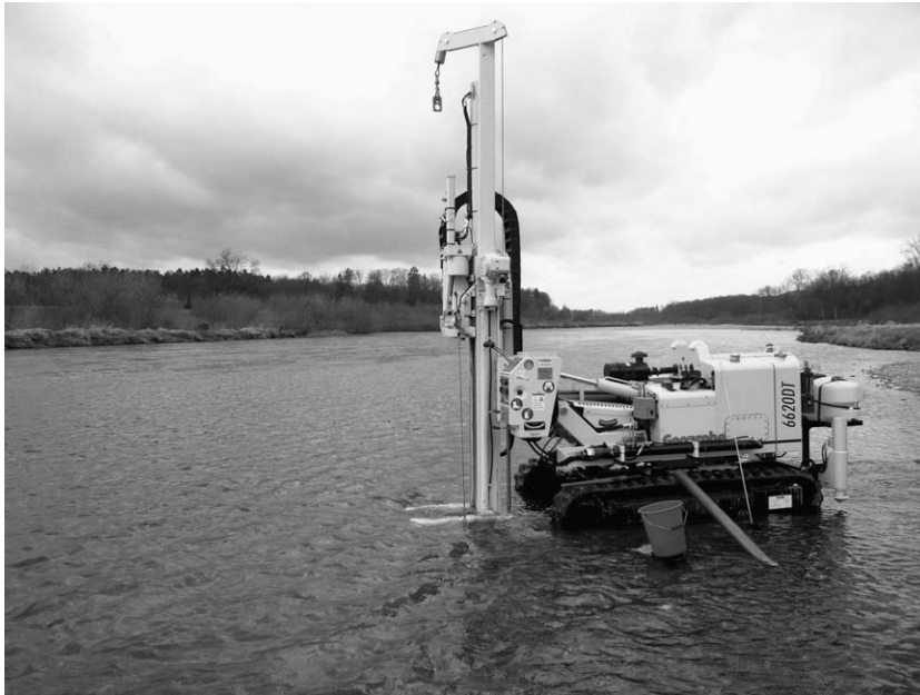
Fig. 3. Photograph of the site showing direct-push installation of the fiber-optic vertical temperature profiler. Viewing direction is downstream.
